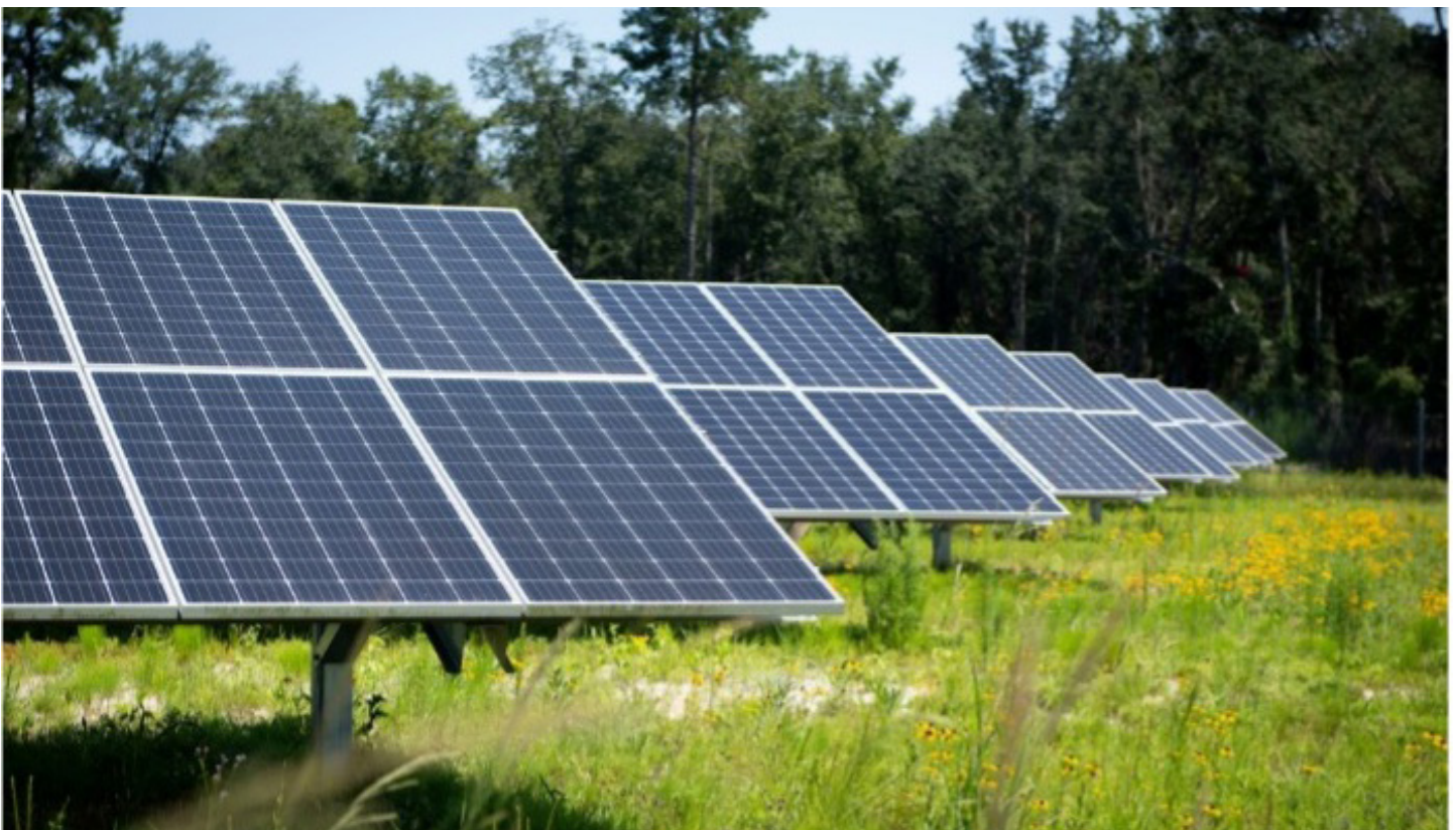
This array of solar panels at Moody Air Force Base, Georgia, saves $700,000 annually. (Department of the Air Force photo by Airman 1st Class Megan Estrada)
